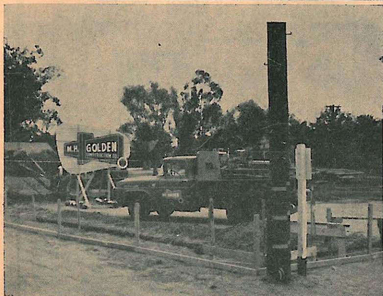
Excavating for foundations for new Alpine Security-First National Bank Building. Alpine Echo Photo
